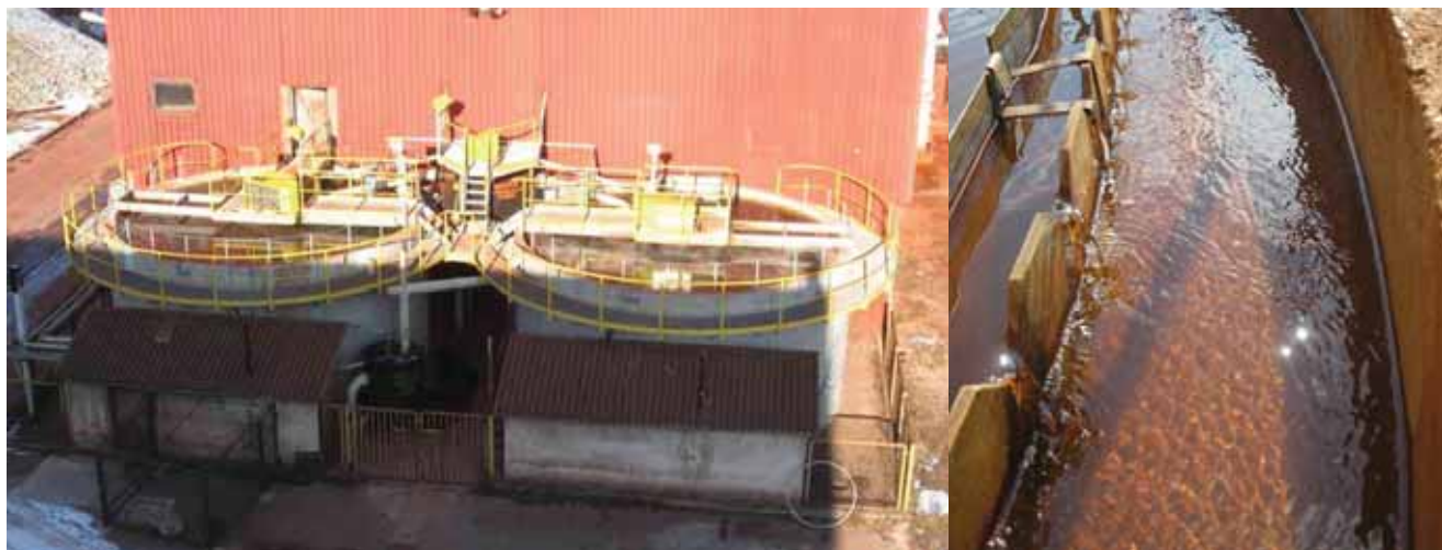
Figure 4: Cooperation between the JSI and ESOTECH: Reconstructed waste-water purification plant in the ACRONI steel works Jesenice (left), outlet of the purified waste water (right).
