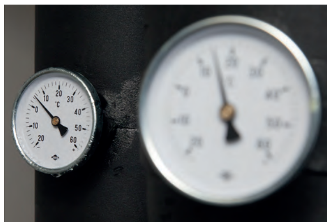
Figure 3: Water-temperature gauges on the cooling-system pipes in the Jožef Stefan Institute Computing Centre at Teslova
