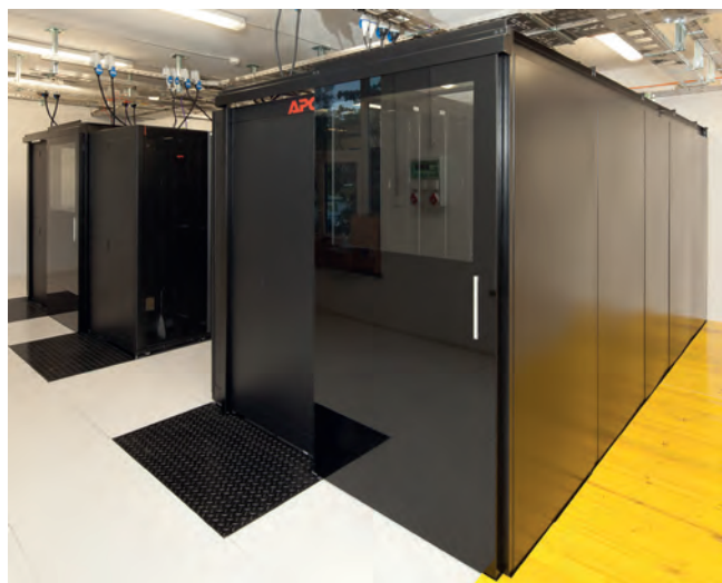
Figure 2: New server racks in the Jožef Stefan Institute Computing Centre at Teslova
